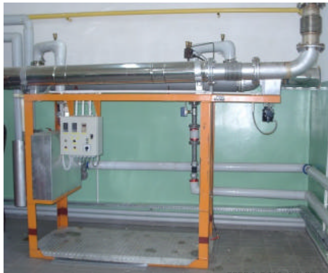
The heat recovery block Photo: W Wdowinski
