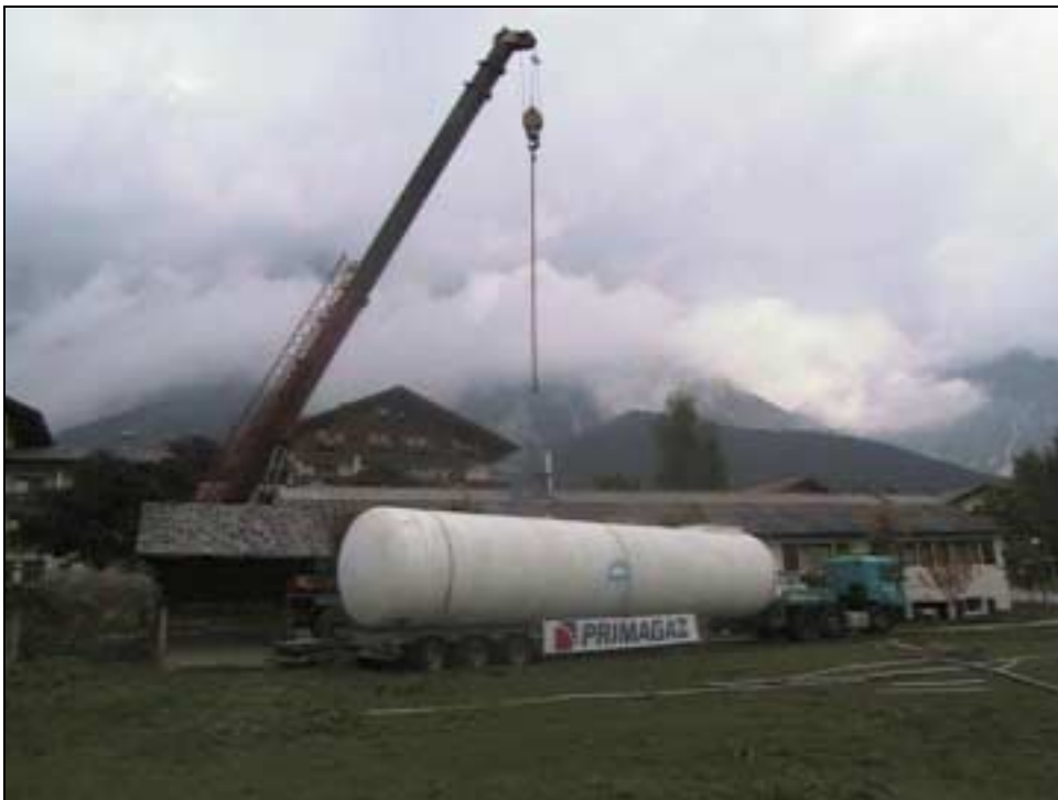
Delivery of tank, Austrian pilot action, hotel Matschner
